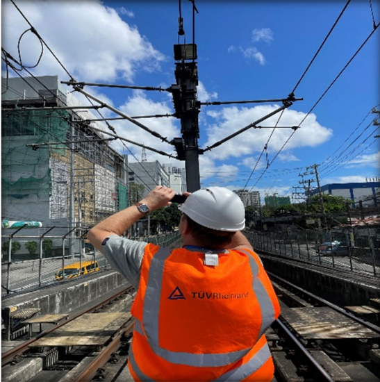
Overhead Catenary System
