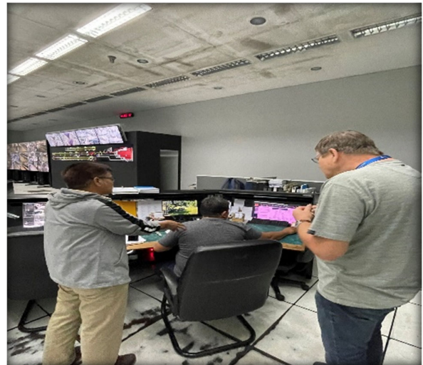
OCC Workstation for SCADA
