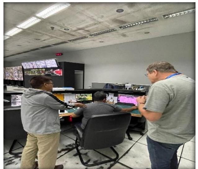
OCC Workstation for SCADA
