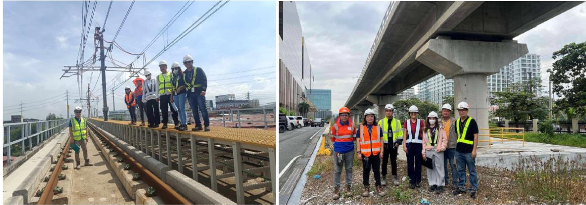
10 September 2024 : Punchlisting Activities conducted by LRTA-PMO, DOTr-PIU, LRMC and EPCC re: Viaduct Structure and Superstructures
